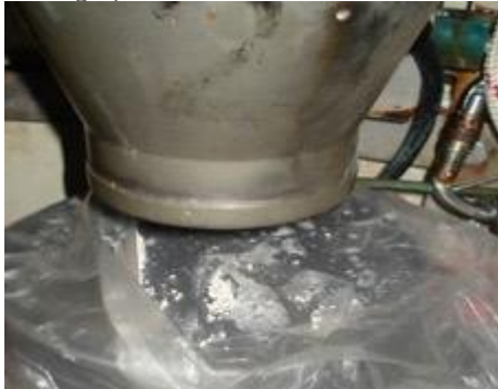
CO 2 particles below scrubber
