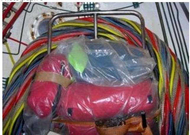
Typical storage of SPs 1 & 2 within a bell
