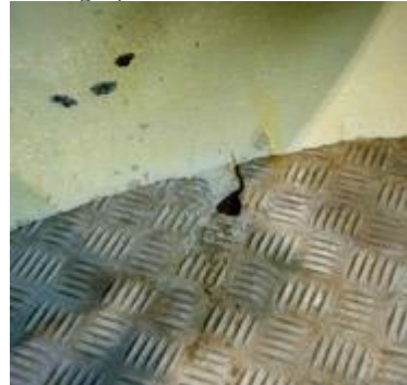
Corroded deck plate below scrubber caused by CO 2 absorbent
