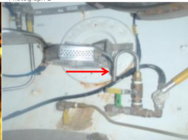
Flood up and 'goose neck' in an old bell. Flood up well below seat level. This has possibly been lowered due to a retro fitted scrubber motor. This change should have been risk assessed.
