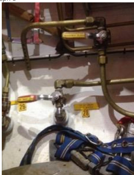
Further example of typical bell flood up arrangement. Flood up depth is below seat height and will not significantly aid the bellman with an incapacitated diver
